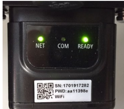
Figure 139 - Irregular communication status between inverter and adapter
